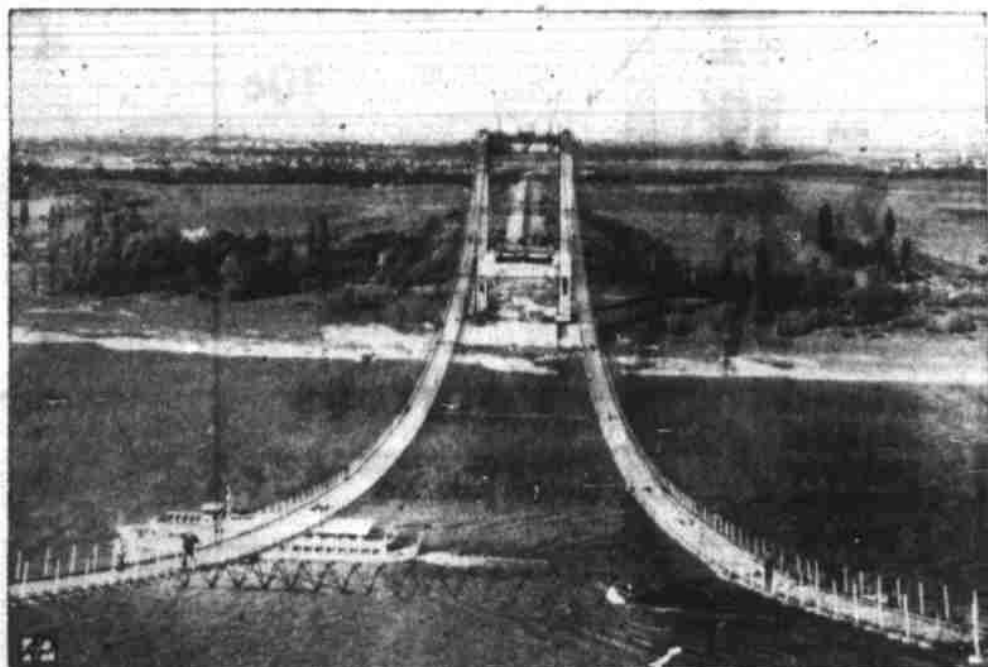
NEW COLOGNE BRIDGE —A partially-completed suspension bridge 1,250 feet long swings above Rhine River at Cologne, Germany. Engineers expect to have it in use next year.
