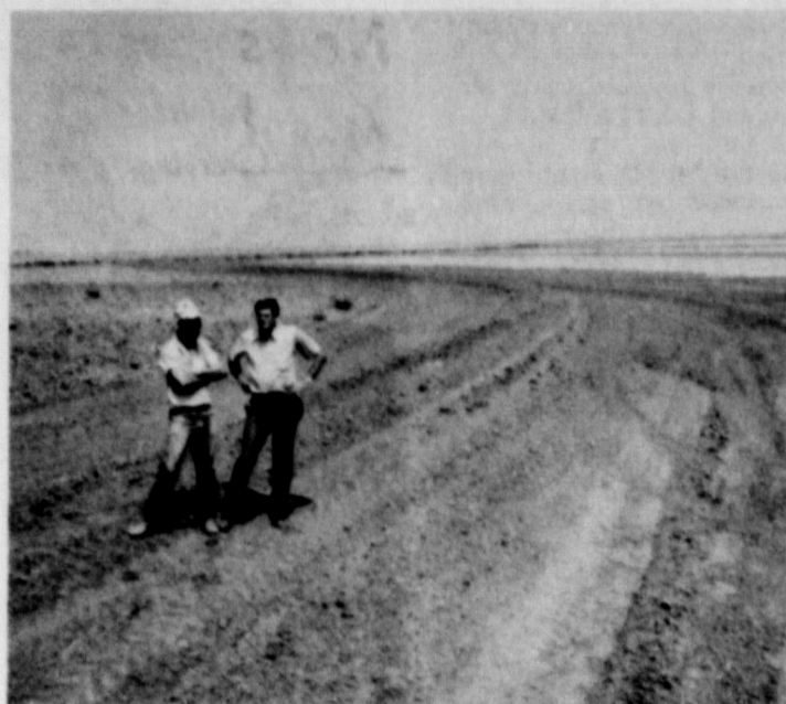
Jim Roach, Conservation Technician, with the Soil Conservation Service and Morris Enloe look over parallel terraces being constructed on the Bill Waters farm south of Grandview. Parallel terraces are being constructed with cost-share assistance under the Great Plains Conservation Program.
