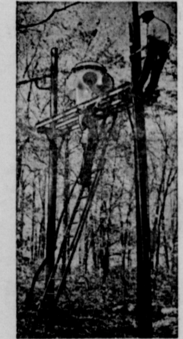
CIVIL DEFENSE siren at Winston-Salem, N. C., is installed by a fire department electrician on the Wake Forest College campus with the assistance and technical advice of Edmund P. Sullivan (on ladder), new city-county deputy CD director. Sullivan's salary is paid 50-50 by Federal and local governments as part of a nation-wide program to strengthen State and local civil defense units. (OCDM Photo)
