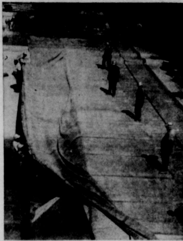
ROLLING OUT THE CARPET —Sixty feet below the surface of the ground in downtown Houston, workers stretch out a Butyl rubber carpet on which the 44-story Humble Oil & Refining Company building will stand when completed in 1962. The Butyl membrane will act as a water barrier for the foundation of the building. This is a unique application of the durable, flexible synthetic which is produced at Humble's Baytown Refinery and is widely used in everything from hot water bottles to conveyor belts, tubing, tires, wading pools, protective clothing for missile launching crews, and car accessories.
