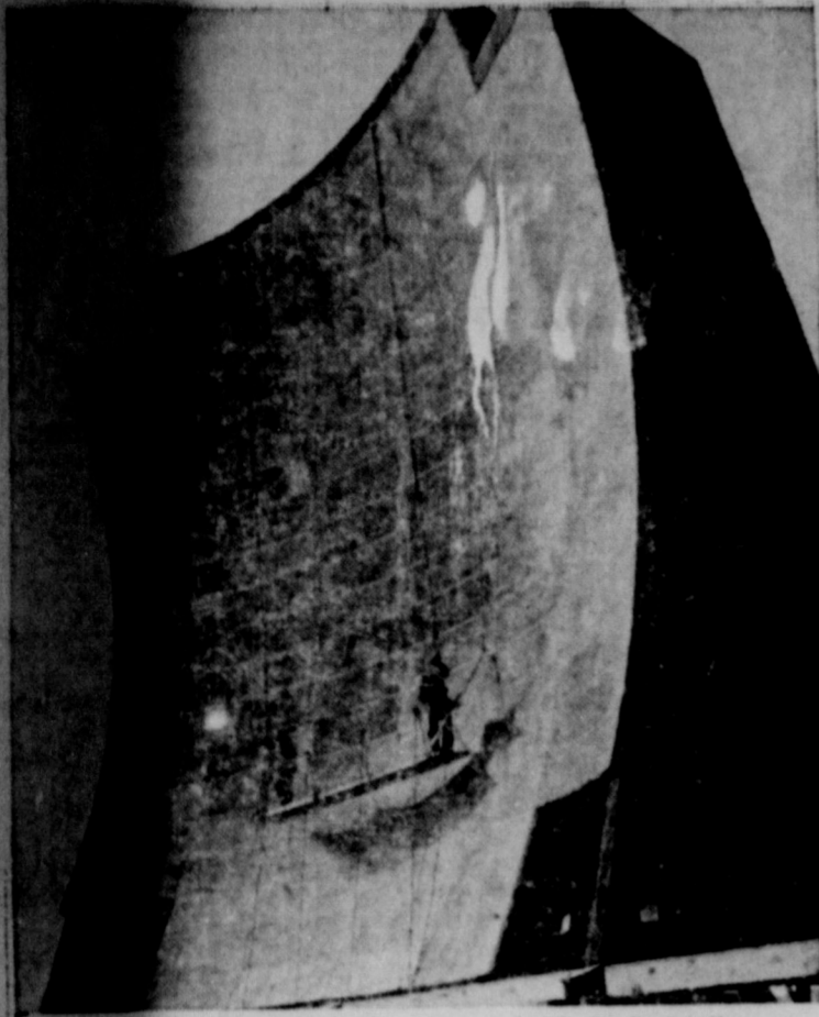
"EAR" DOCTORS —Calking seams of this 60-foot-tall parabolic antenna is an annual chore for technicians who work on Alaska's "White Alice" communications system. The giant "iron ear" is one of many along a 3,100-mile line that serves civilians, commercial and military purposes.
