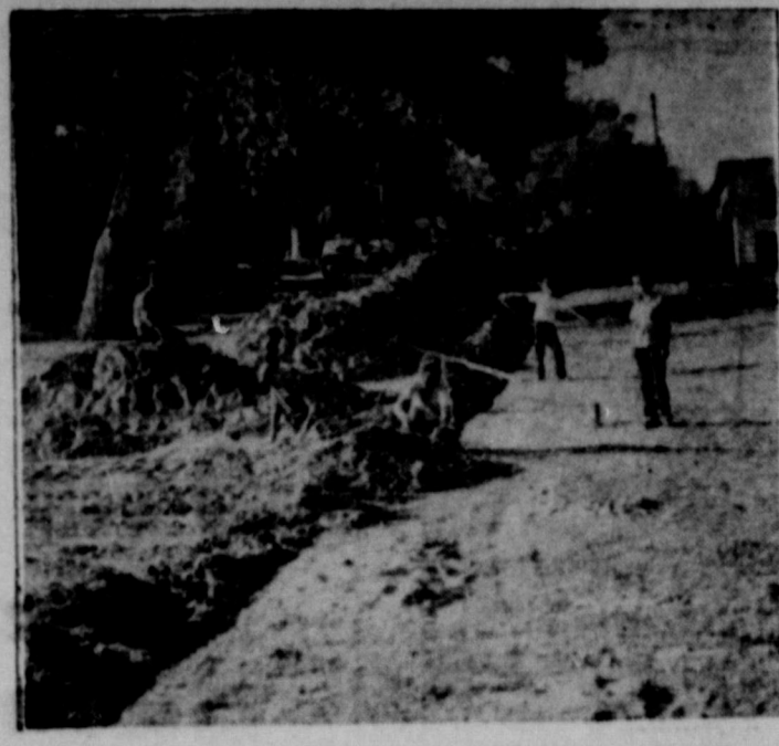
Boys' Ranchers lay 8" tile which connects the 26 buildings at America's first Boys Ranch, Amarillo, to a central disposal unit. The new system will eliminate the many septic tanks at the Ranch which require frequent cleaning and will provide for future buildings.
