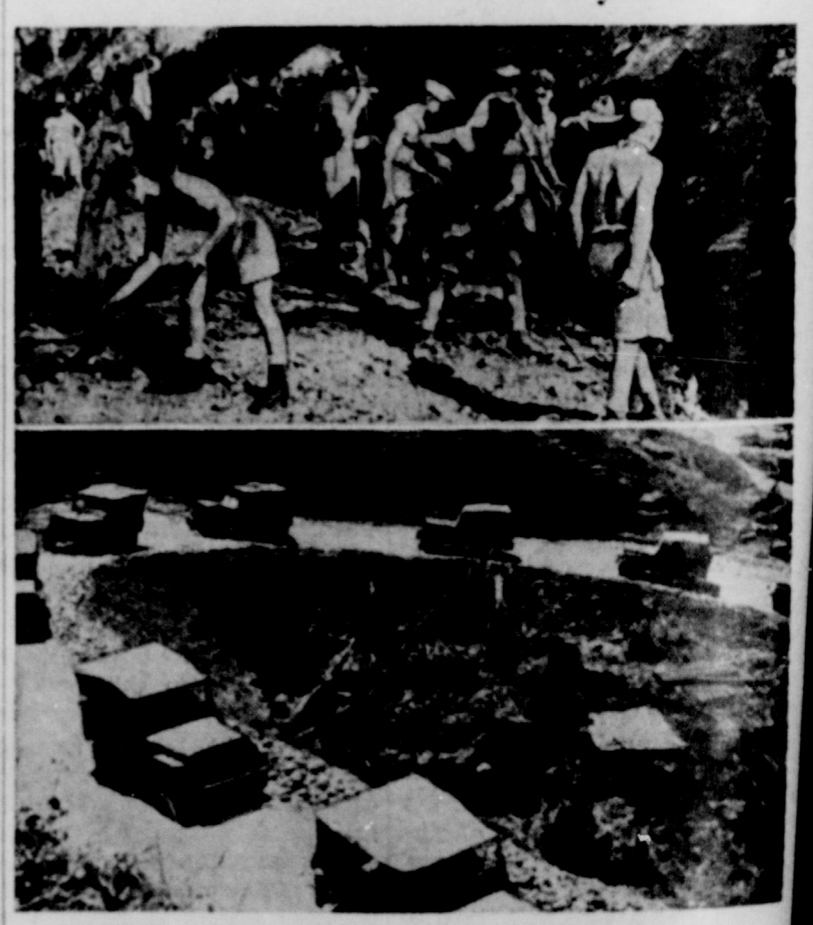
British engineers in Burma are hacking highways through jungles, mountains, to create a system of roads and supply lines over which they plan to force the Japanese from their positions in that sector. At top, British troops are working on a new stretch of road. Below: A convoy of jeeps carry supplies around a loop on a new road in Burma.
