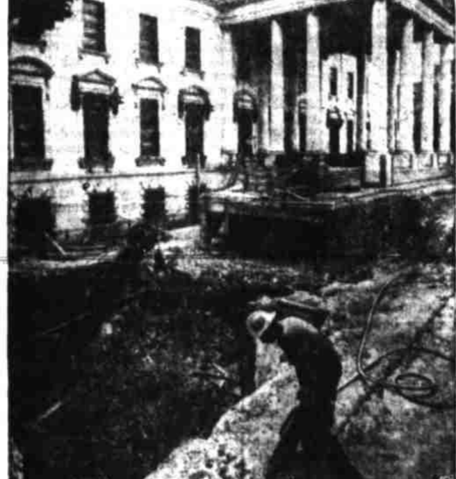
REMODELING THE WHITE HOUSE —A workman operates a jackhammer during remodeling of the White House in Washington, scheduled to cost $4,500,000.
