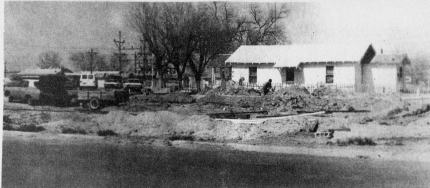
NEW LAUNDRY SITE . . . B.V. Hughes of Farwell is constructing a coin-operated laundry in Mulshoe at the corner of Fourth Street and Ave. E. Hughes stated that the laundry will feature 36 washers and 16 dryers and will possibly be completed in two months. The cost of the project is estimated at $30,000.
