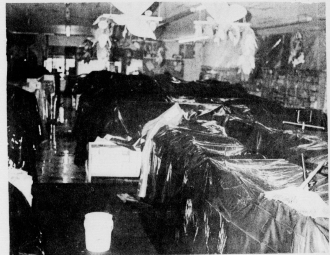
RAIN CAUSES PROBLEMS . . . Due to their roof being partially off, the C.R. Anthony Store in Muleshoe was flooded Thursday during the heavy rains that fell. Assistant Manager Gerald Carnes reported that roofers who were re-roofing the store had the roof partially off when the rain started, flooding the store. He said that they were inventorying the damage Friday. Due to the water, the store was closed Friday and Saturday, but re-opened Saturday.
