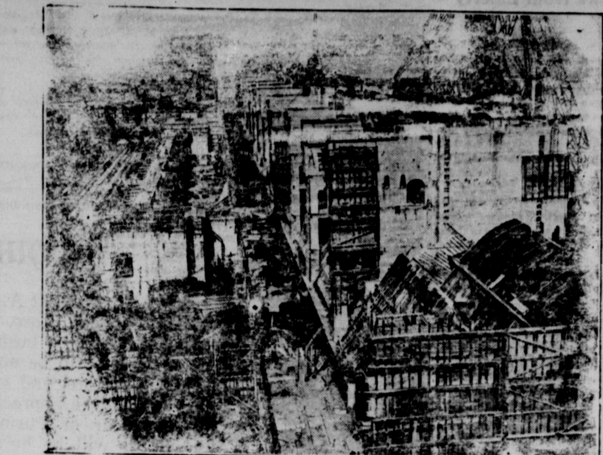
General view of the construction work at Wilson Dam, Muscle Shoals power plant.
