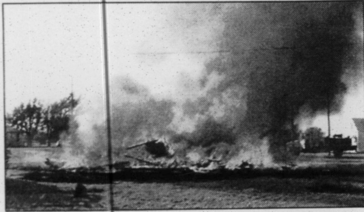
"Who has the marshmallows?" was just one of the many comments heard when local fire fighter use a condemned house as a training drill Saturday. This old house on the corner of 1st and Collier was in need of tearing down. This lot will now be given to the Groom Economic Development Corporation for development.
