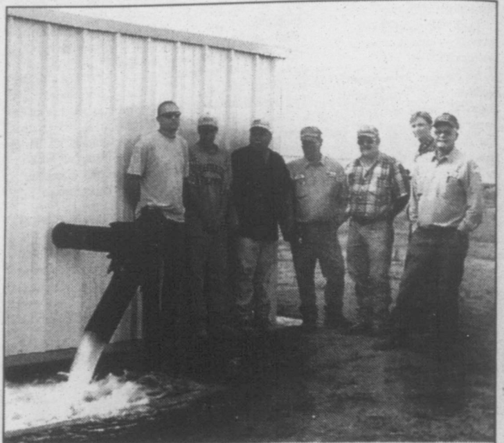
Some very happy guys turn on the faucet at the long waited for new well. For 5 years, Mayor Joe Homer, City Employees Donnie Evans and Louis Leven, Brandt Engineering employee Justin Search have been working to get the well going. representatives of Fuller Construction, Tom Hilleary, Josh Hilleary and Larry Roberts came on board in the later phases of the project but were glad to see it completed.
