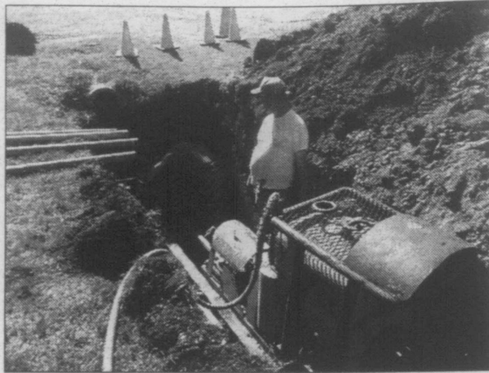
New pipe is being laid between the new water well and the water tower.
