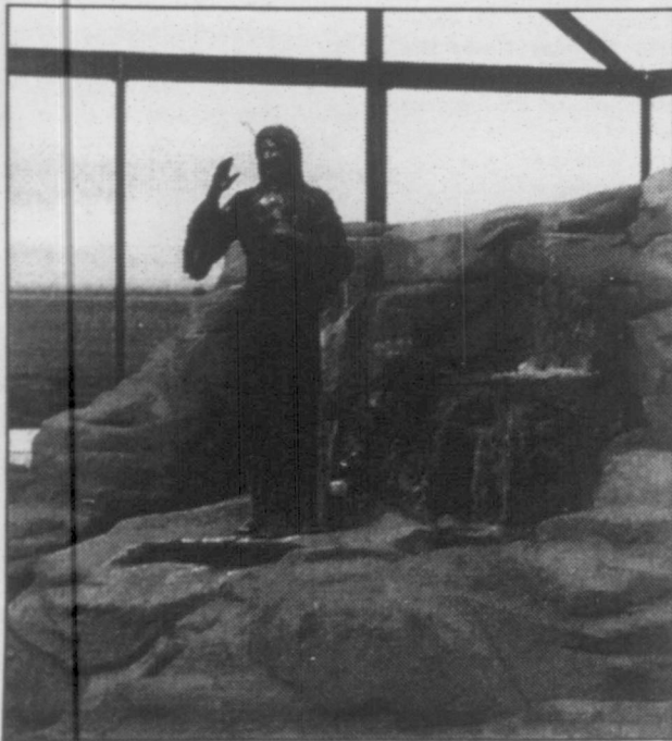
Work is continuing at the Cross of Our Lord Jesus Christ. A new building is going up around this lovely fountain.
