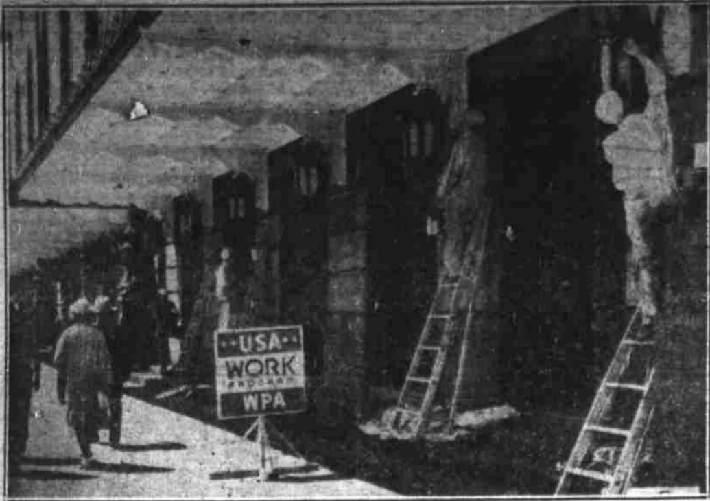
The site of the national Republican convention at Cleveland was refurbished inside and out for the event at a cost of more than $300,000, mostly from federal relief funds. WPA signs were greatly in evidence as workmen put the final coat of paint on the marquee. (Associated Press Photo)
