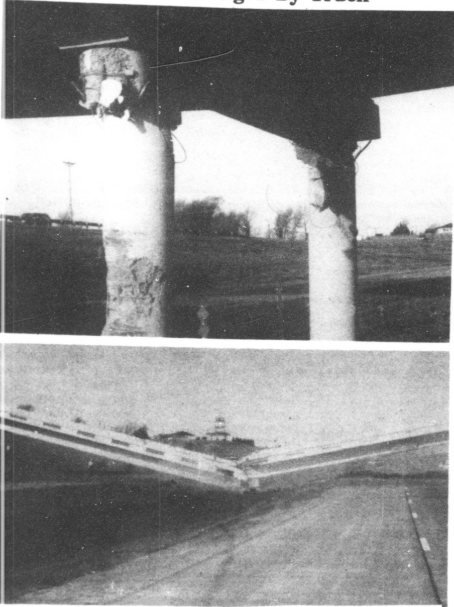
↓ ALANREED BRIDGE IS FALLING DOWN MY FAIR LADY ↓ Alanreed was the scene of a tractor trailer accident recently in which an overpass bridge was destroyed. The rig driven by Albert Blakley was westbound when it crossed the road and crashed into two pylons of the overpass at I-40 and FM 291. The bridge will have to be completely demolished. For several days I-40 was re-routed, while highway department employees worked to clear the wreckage. Eastbound I-40 is now reopened. Westbound should reopen soon.
