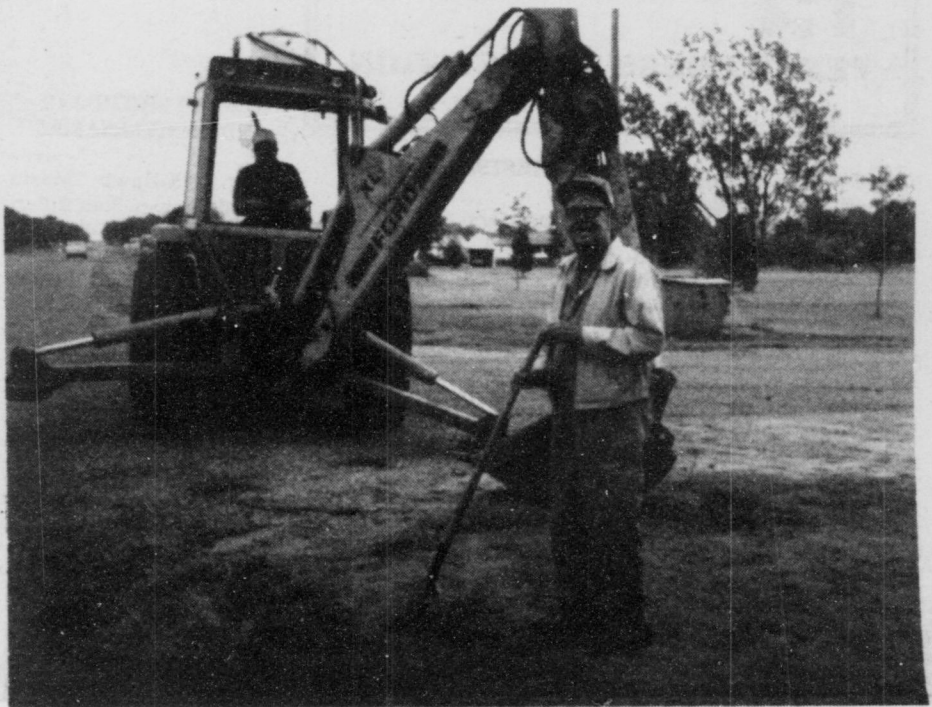
Al Homer breaks the ground as work begins on the water system.
