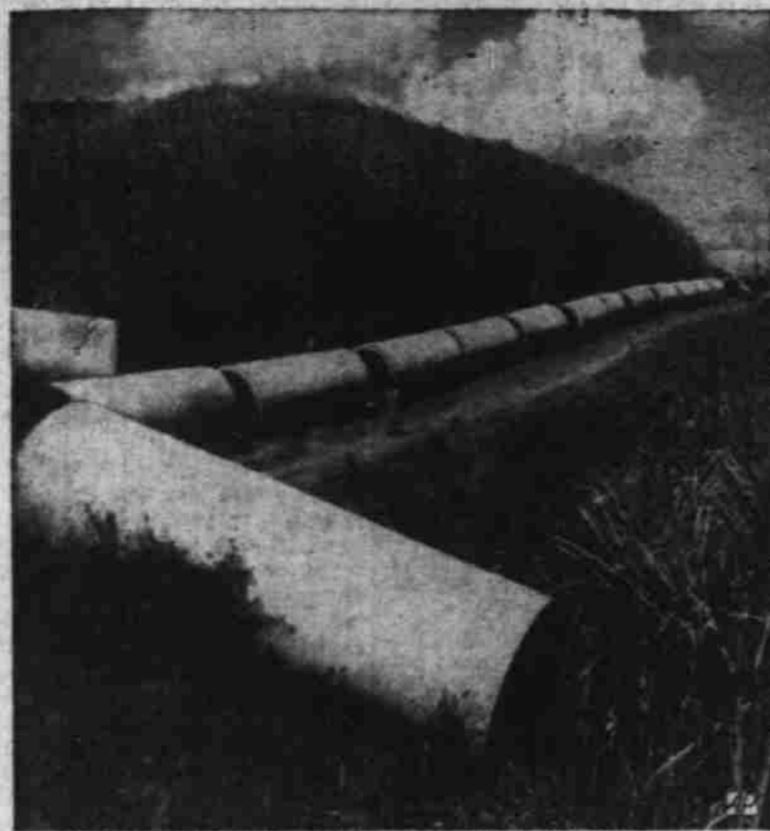
PUERTO RICO'S 'LITTLE INCH' — Sections of Puerto Rico's "Little Inch", $25,000,000 San Juan water system, line the route from filtration plant to the reservoir.
