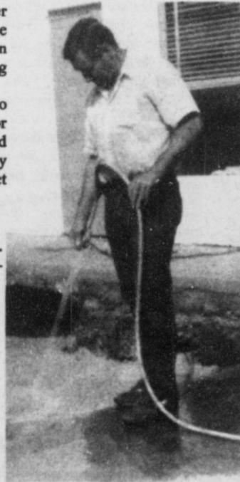
Pav Pavlovsky worked diligently this past week removing and placing new gas tanks at Pav's Station.
