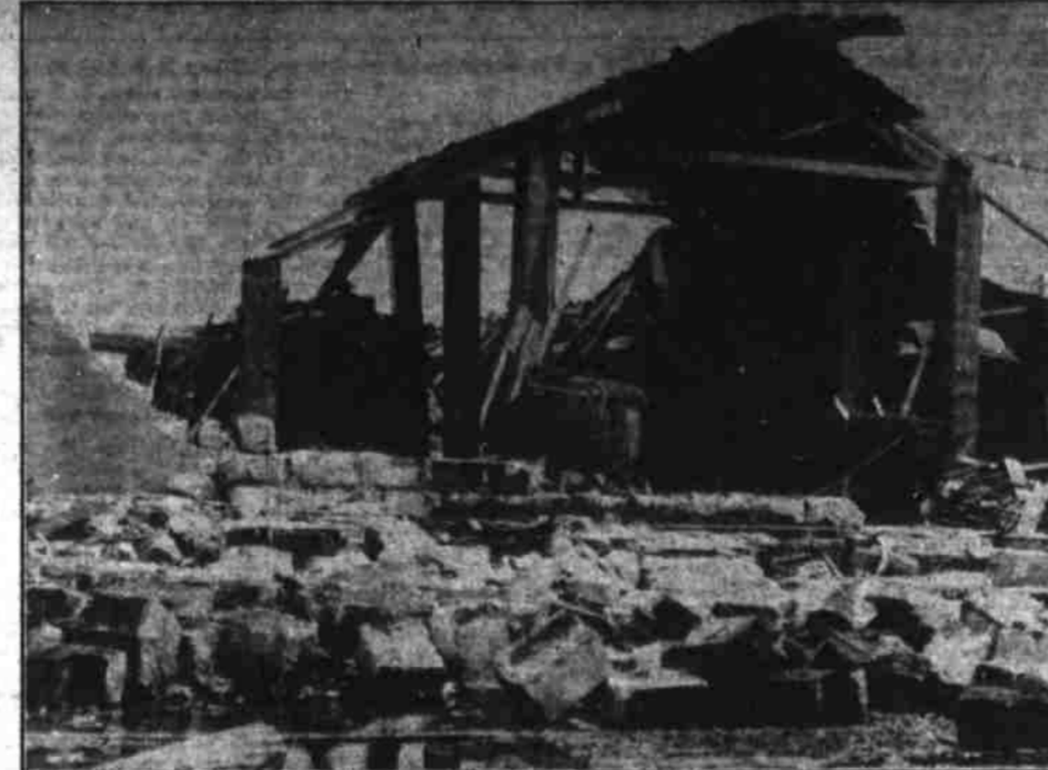
This picture shows a heavy building wrecked by the tropical hurricane which struck with intensity at Gardena, Cuba, killing 30 persons, injuring 100 others and wrecking 2,000 houses. Damage was unofficially estimated at $6,000,000. (Associated Press Photo)
