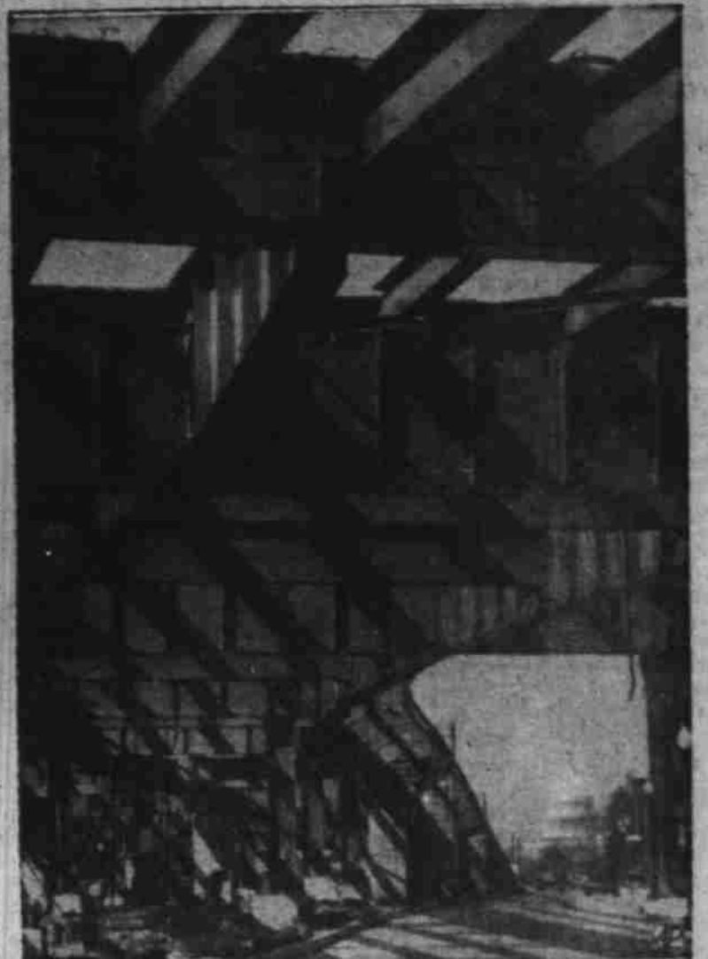
STEEL FRAME —The Capitol at Washington stands framed by the steelwork for the new South Capitol Street bridge which will span the Anacostia River in November.
