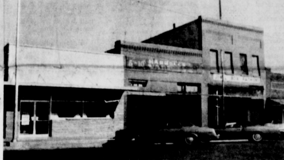
Work began this week on the first stages of remodeling the American National Bank building by Wiley Hicks Construction Co. of Amarillo. Projected completion date is November 1. (Staff Photo by Linda Haynes)
