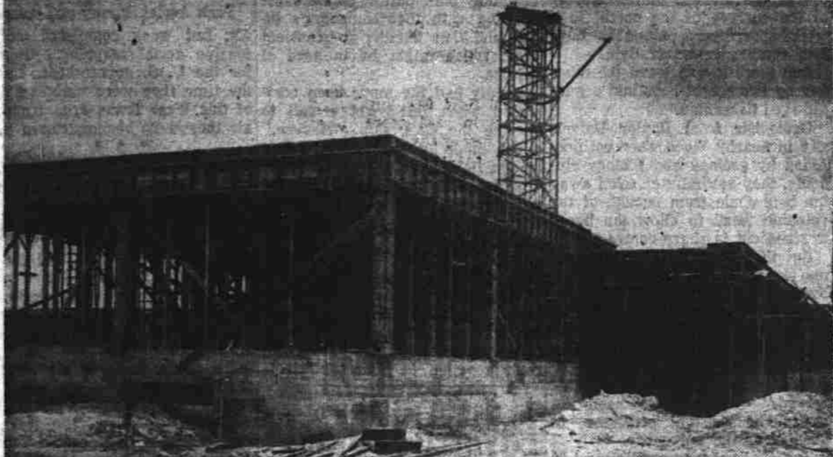
HOSPITAL JOB PROGRESSES — Workers toil at preparing footings for a section on the south end of the Veterans Administration hospital here as others install forms for first floor columns on the northern section in the background. The men are mostly at basement level, but others may be seen descending into holes for footings. These are sunk to a depth of 24 feet and are dug by hand. Below, the concrete for the laundry wing, on the extreme north end of the building, is poured. This view is taken from the northwest and looking to the southeast. At the point where the scaffolding rises, the main portion of the building will tower for six stories. (Jack M. Haynes Photos).
