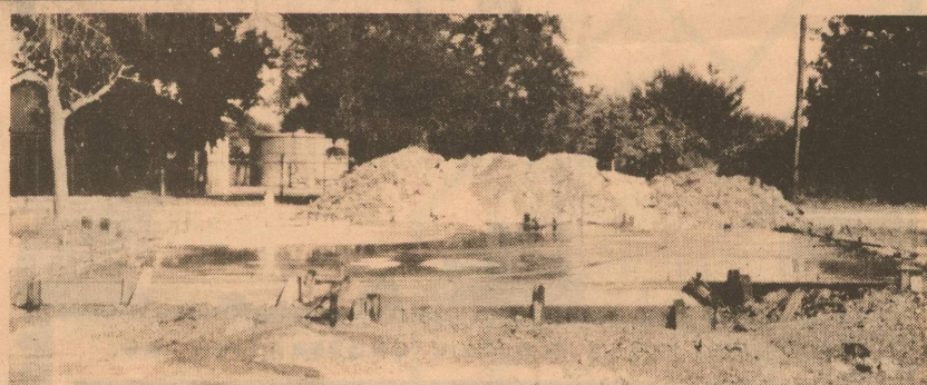
Pictured above is the future site of the new Senior Citizens center located on the corner of Gillis and Poplar. The land was donated by the City of Eldorado.
