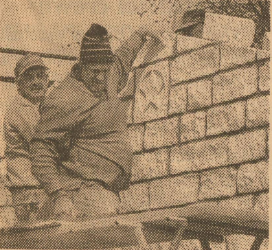
Stone masons Aaron Lankford and Bill O'Neal from San Angelo put the finishing touches on the tone facade at City Hall.
