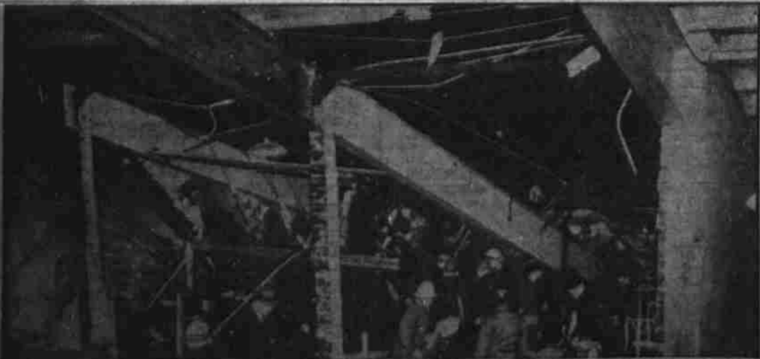
Police and firemen are shown inspecting ruins in the Cleveland stadium, following an explosion that injured four and endangered 200 Great Lakes Exposition employees and concessioners. Damage was estimated at approximately $25,000. (Associated Press Photo)
