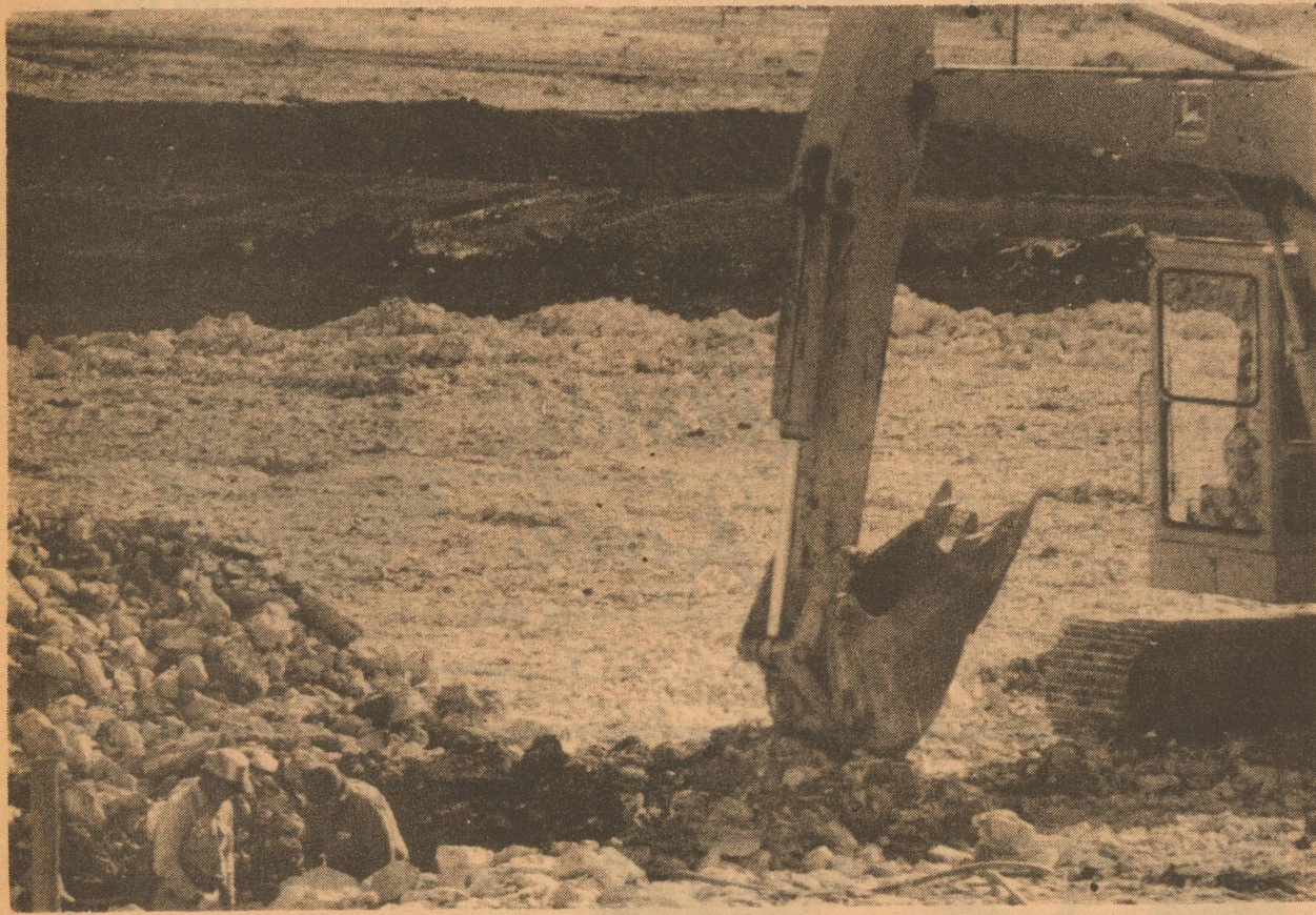
Progress is somewhat slower than expected on the sewer plant project according to City officials. The
