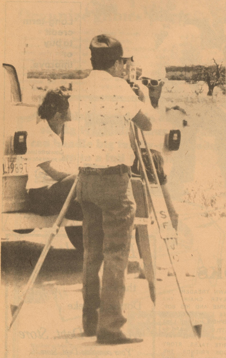
Surveyors were the first evidence of Eldorado's soon to be new sewer system.
