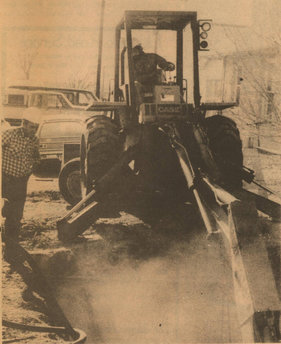
GTE has contracted Burnup & Sims to dig 11 conduits for telephone cables for future growth. Pictured here is Ronald Sturn looking into the deep manhole while Jesus Fuentes is operating the air-drive backhoe.
