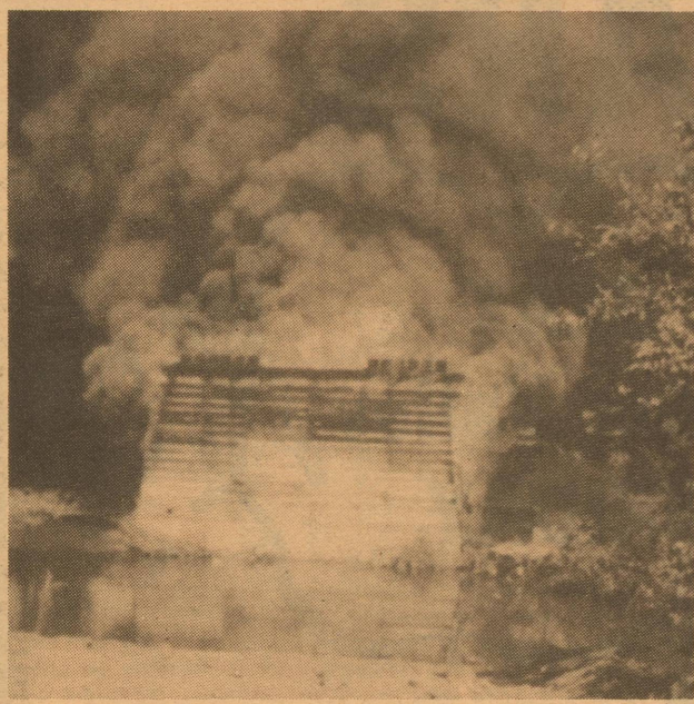
RAILROAD FIRE — The last section of a railroad bridge in Christoval went up in smoke Saturday while a demolition crew worked to tear it apart. The fire started when a bolt heated by a cutting torch fell on dry timber. This picture was taken by Travis Parker who watched construction of the bridge during the 1920's and then watched it burn Saturday. The Christoval fire truck was on hand in case a grass fire started from this fire.
