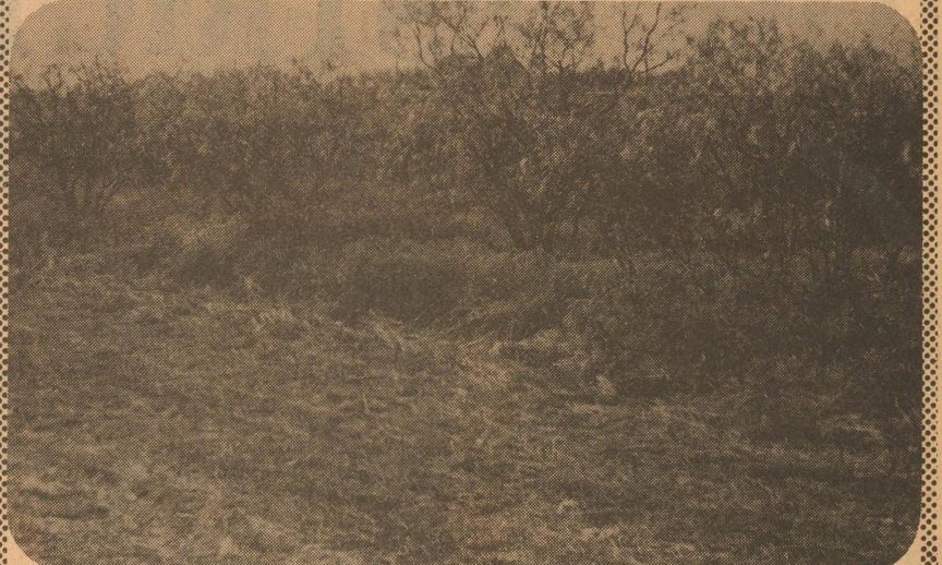
For a week, this Block in south Eldorado has had heavy equipment clearing the brush away. See the final results of the construction on page 6.
