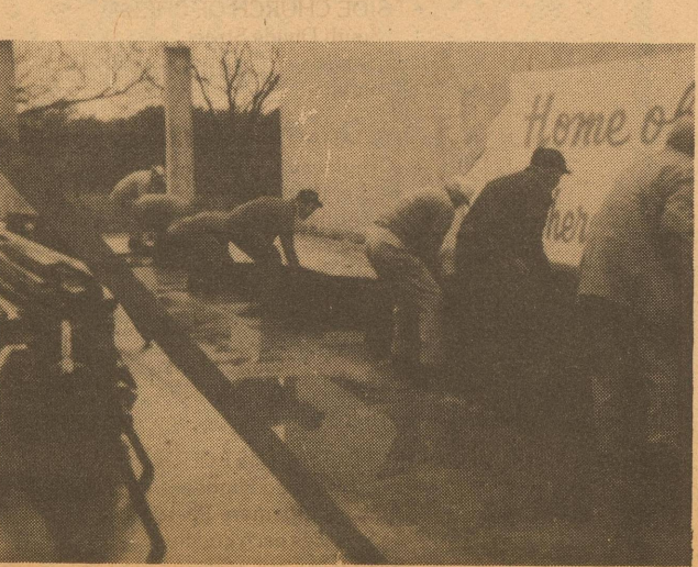
Sixty feet of wall went up with the help of Zach Tounget, Sid Johnson, Pete McBurnett, Ken Tounget, Sid Shipley, Pate Boone, and Sunny Stigler. Christoval's Community Building is becoming a reality.
