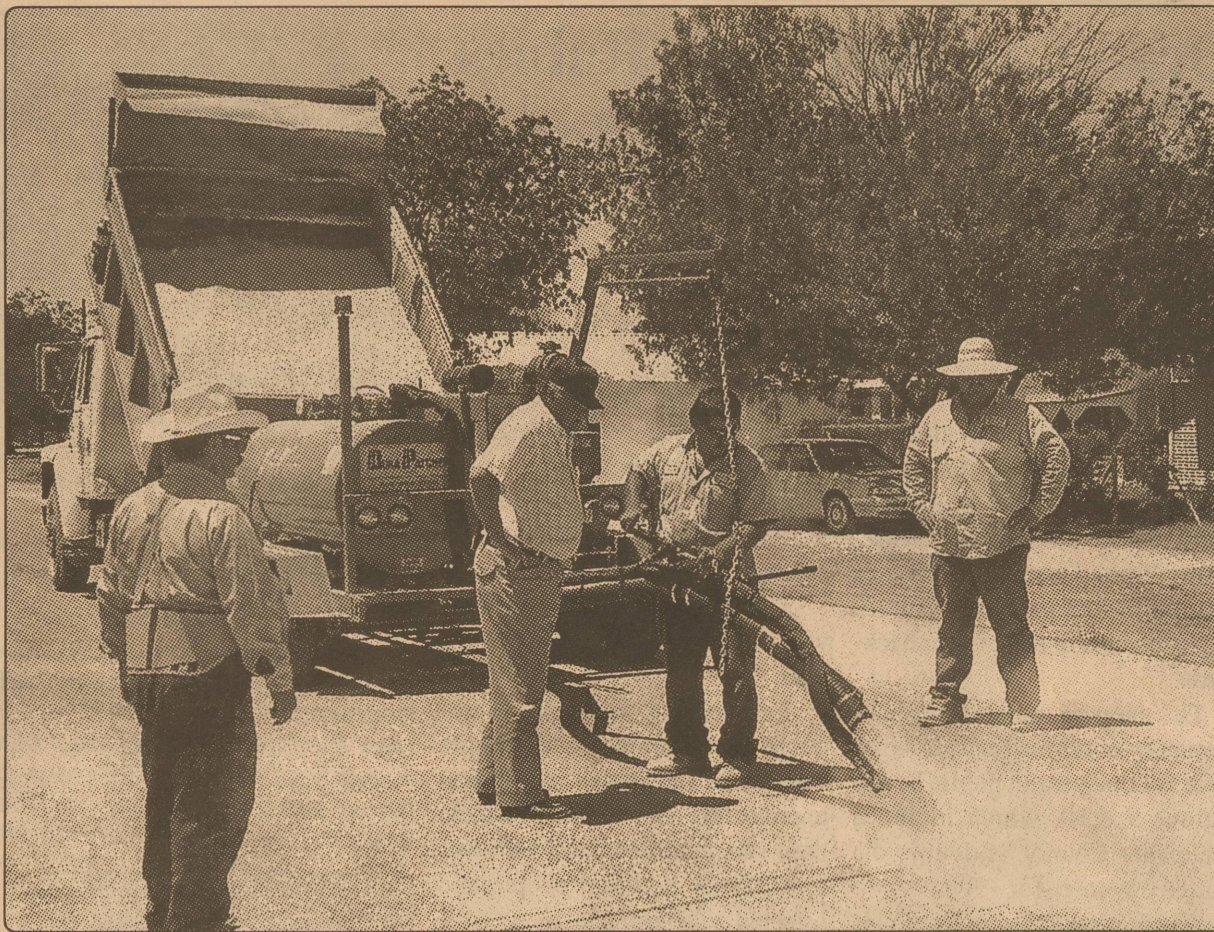
Pothole patchin' — City crews received instruction recently on operation of the City's new pothole patching machine. The machine was put into service last week and should be running throughout the summer.
