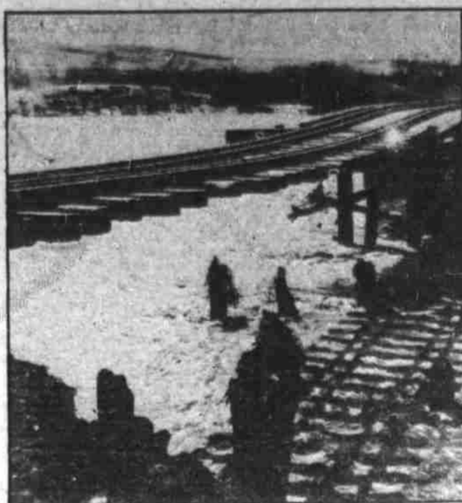
Torrential rains, bringing floods in some sections, washed the debris of dust storms from many parts of Nebraska, Kansas and other drought-stricken states. Above is shown a bridge near Ord, Neb., with many of its supports swept away by the bank-full torrent. (Associated Press Photo)
