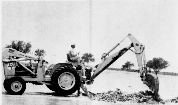
DITCHING WATER -- Water came down Blackwater Draw about mid-morning Friday following Thursday's heavy rains. Shown here is a city employee cutting a ditch across South Main Street to channel the water into open country. The water flooded several homes and businesses before it receded.
