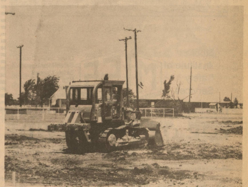
County equipment pulls up stumps and roots and prepares the ground for the new ball field in the Schleicher County Park.
