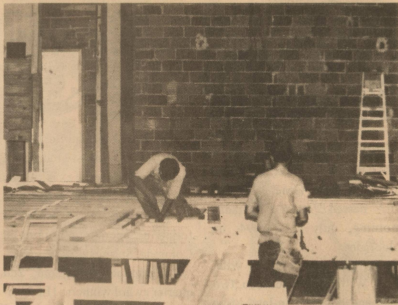
Shown above are Richard Menendez (R) and Herman Walker (L) as they work to enlarge the stage in the Tom Ratliff Civic Theater. The work is part of phase one of the theater restoration.
