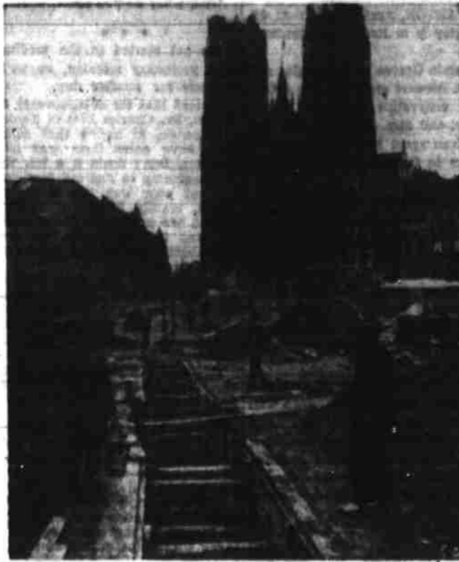
BRUSSELS BUILDS SUBWAY — Hole in the ground in front of St. Gudule Cathedral, Brussels, Belgium, is part of 40-year subway project scheduled to be completed in 1951.
