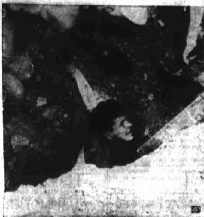
RESCUED FROM CAVEIN —Rescuers aid Harold G. McCormick, 24-year-old college student, shown trapped in a sewer ditch he was digging in Endicott, N. Y. Heavy gravel pins him down. Fellow workmen on a housing project eased him to a standing position by pulling on a sheet they wrapped around his chest. They dug him clear in one hour, 50 minutes. He suffered no apparent injuries. (AP Wirephoto).
