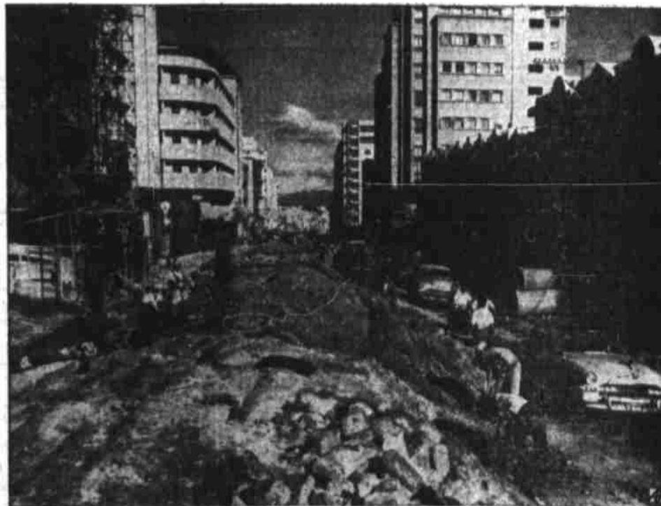
CONFUSION BEFORE CONTROL — A Caracas street presents a confused scene as construction is under way to further a traffic control plan in the Venezuelan capital.
