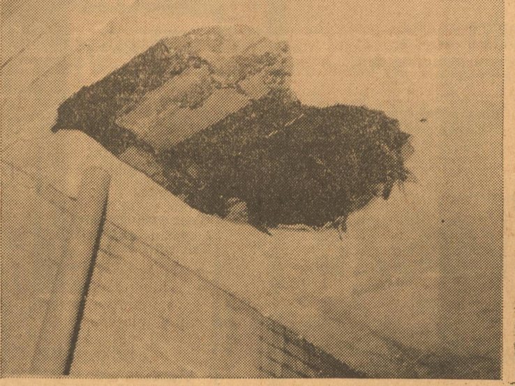
Hole In Hallway Ceiling About 3 Years Old
