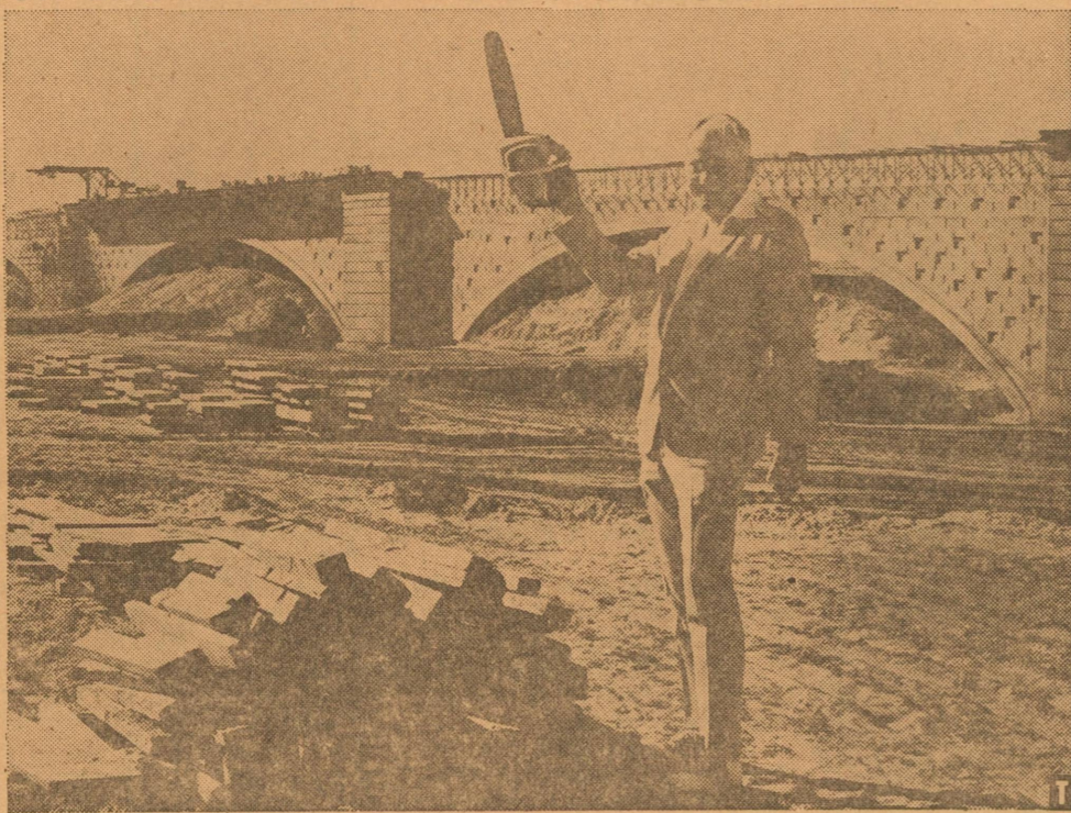
Robert P. McCulloch, Sr., president of McCulloch Corporation, one of the world's largest manufacturers of chain saws, stands in front of the London Bridge, which is being reconstructed at the Arizona resort town of Lake Havasu City. He holds a Mini-Mac 6, the lightest chain saw made. The company's saws were used in the reconstruction of the bridge, the largest antique an American tourist has ever brought back from Europe.
