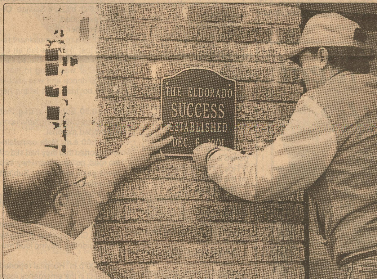
Just a little to the right — Joey Jones (right) assisted Success publisher Randy Mankin Monday. The men installed a plaque on the front wall of The Eldorado Success office commemorating the founding of the newspaper 100th ago.
