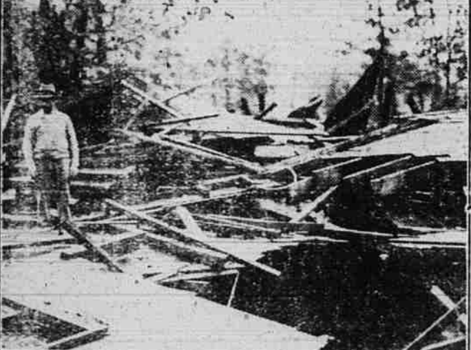
More than 50 persons were injured in a gale that lashed Long Island causing thousands of dollars worth of property damage. Twenty cottages were blown into Jamaica bay. Above picture shows a bungalow toppled over by the storm at Broad Channel, Queens. Wreckage of a two-story building at Merrick, L. I., is shown below. (Associated Press Photos)
