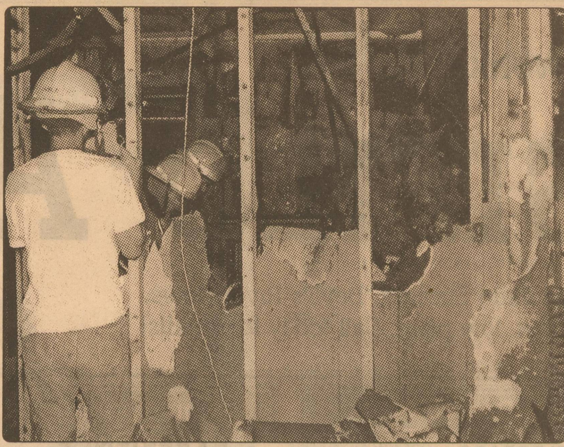
Making sure it's out — Firemen worked their way through a burned out apartment on North Street last Friday, looking for hot spots. The fire gutted one apartment and caused heavy smoke and water damage to three others. (see story on Page 1)
