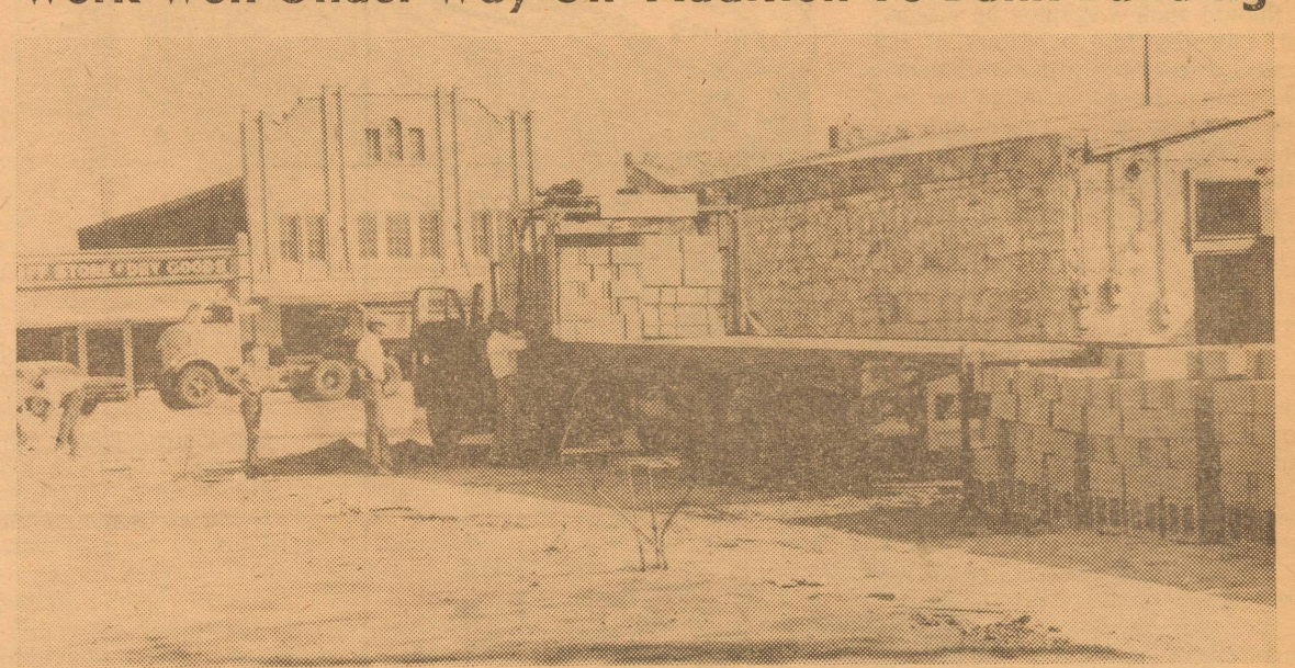
THIS PHOTO taken last week shows cement tile being unloaded north of the First National Bank building. Since then, the walls have been erected for the addition to the bank which will include a drive-in window.
